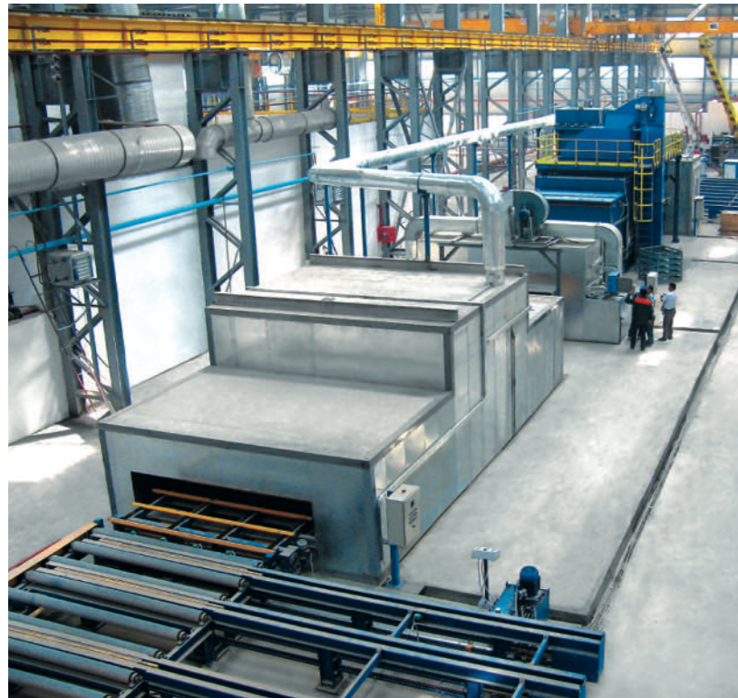
Shot blasting and preservation line for metal-roll
